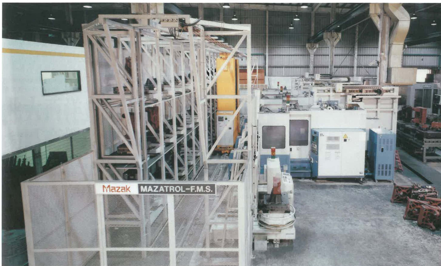
Companies that manufacture or source in the region are capitalising on lower prices and labour costs. (Photo courtesy of Chen Hsong).
